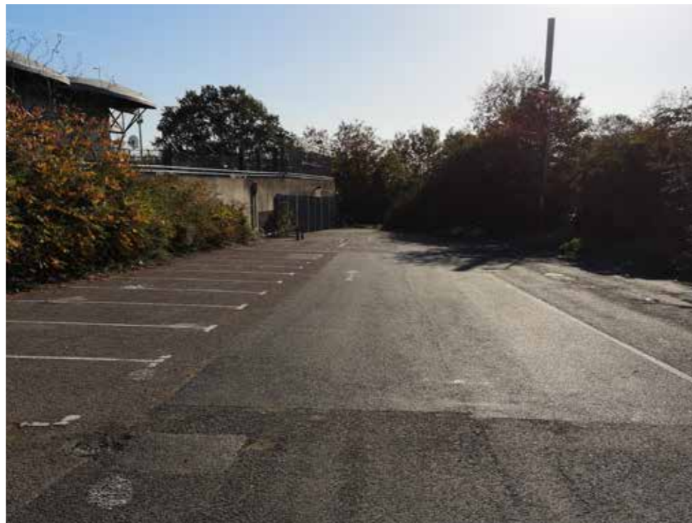
Access Road to Secured Car Park in the South. Retaining Wall on the Left
