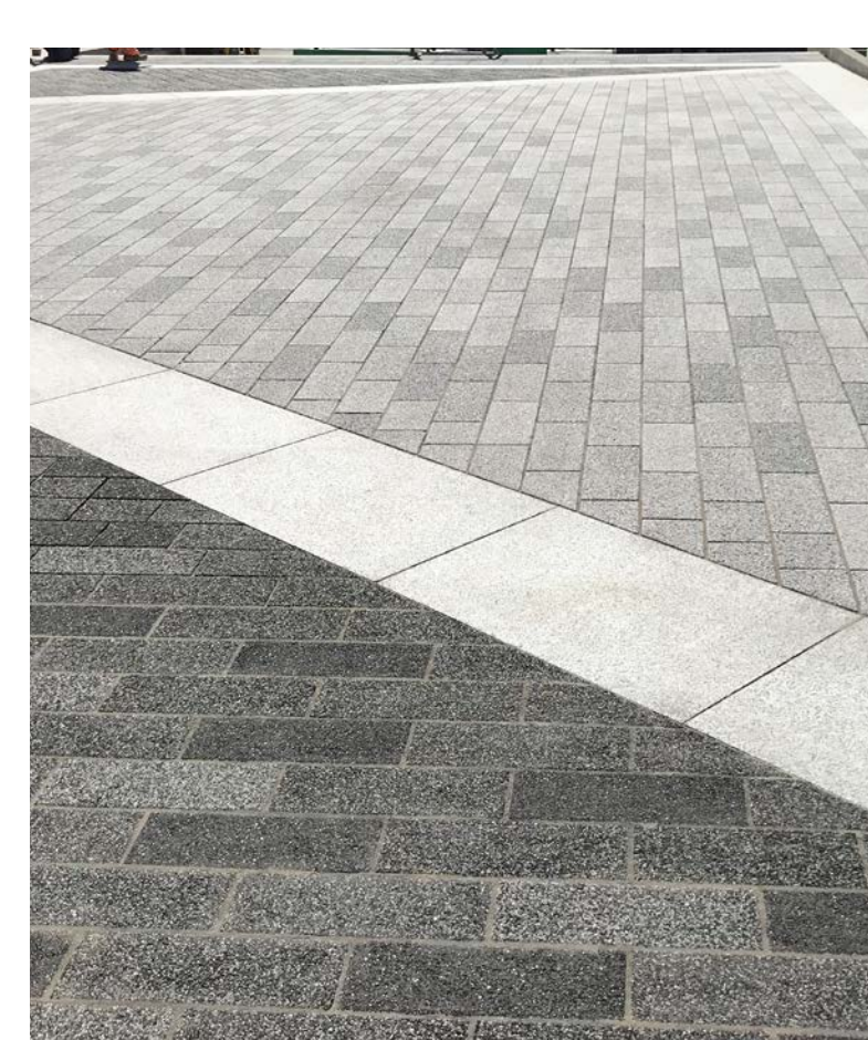
Continuous high quality paving finish incorporating robust mixed tone block paving and stone banding
